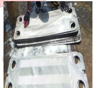
Cleaning of HT Plates
